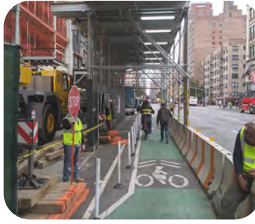
Poor Construction Right of Way
